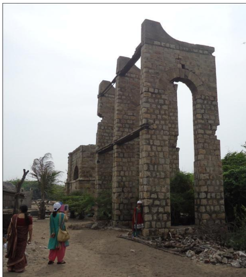
Fig.4: Remains of Overhead water tank structure
