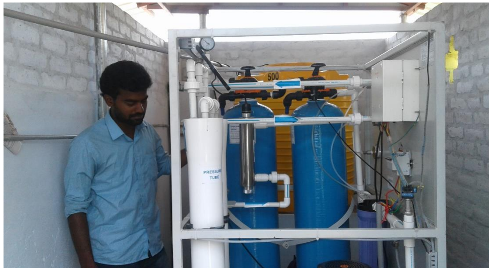
Shri. Nagur Meran, Supervisor of the supplier (Eureka Forbes) carrying out regular maintenance of the plant for proper quality
